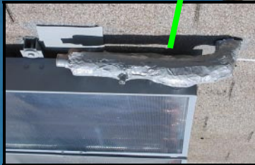
Finished return assembly with Insulation, aluminum tape and matching paint (Picture shown from top view looking down)
